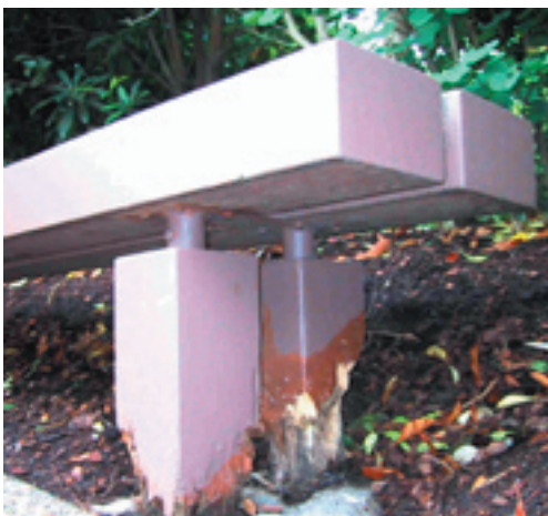
Rotting seat posts made from untreated timber
