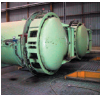
Modern, covered treatment plants showing cylinders and charge of timber ready for treatment . (Photographs courtesy Harry Greaves)
