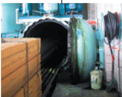
A typical timber treatment process for posts, power poles, landscaping logs and the like.
